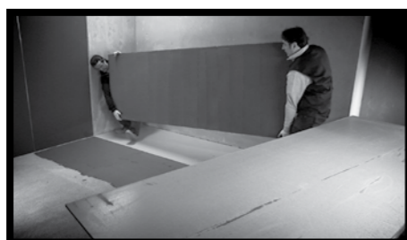
Fig.58 - 1 -To handle slabs, raise them to their upright position, whilst grasping them from the top edge. Move the slab keeping it straight and with the aid of another person.
